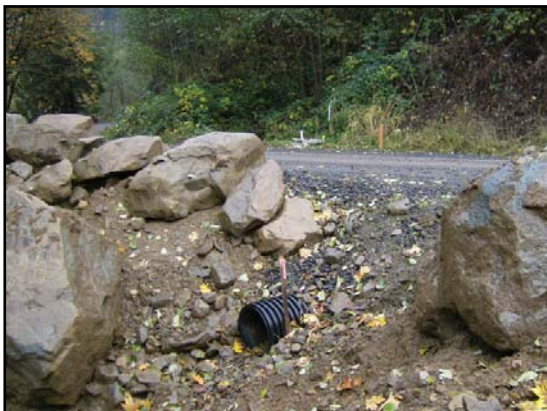
Cross-drain culvert on Dellwood Mainline, Weyerhaeuser
