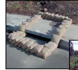
Sand bags around drain inlets to prevent sediment from reaching storm drains
