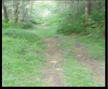
Weyerhaeuser road decommission to help prevent long term culvert failure and road washout.
