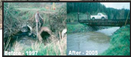
Blocked culverts replaced with a railcar bridge to allow water to flow freely.
